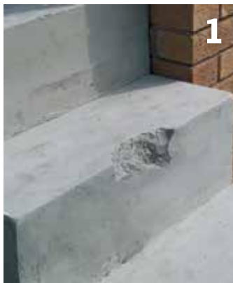
Broken nosing on external step
